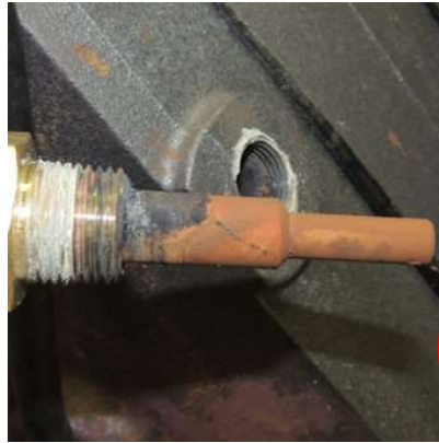
LWCO Probe fouled
