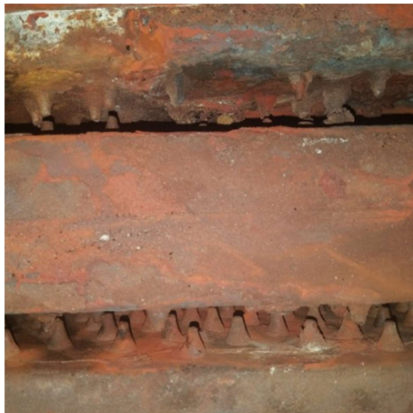
Corrosion above the waterline
